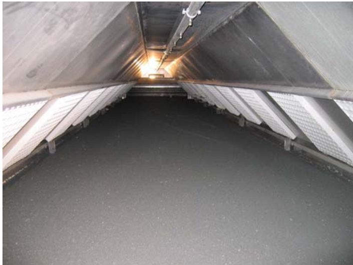
Photo 1: Interior view of the belt dryer with sludge.
